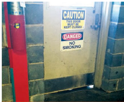
A typical single-swing door. The sign says one thing; the gap, bottom right, another
