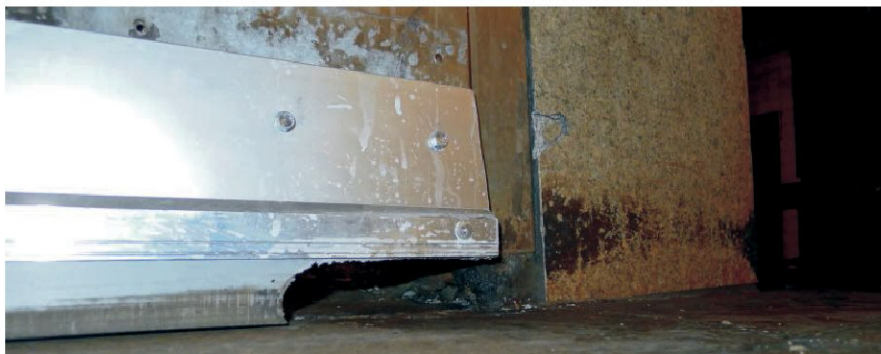
The grey vinyl strip on the base of this door is a weather strip. Note how the rodents were able to easily gnaw through it (also note the tooth marks in the vinyl)
